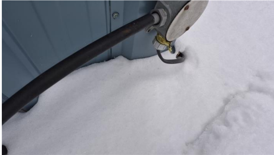
Photo 17: Municipal Garage – Existing Unprotected Power Cabling at Ground Level
