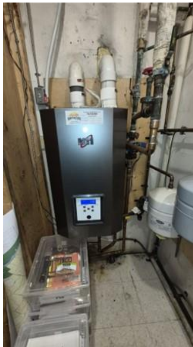
Photo 14: Recreation Hall – Heating and Domestic Water Boiler
