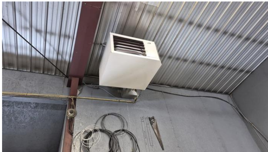
Photo 16: Municipal Garage – Existing Newer Garage Area Unit Heater
