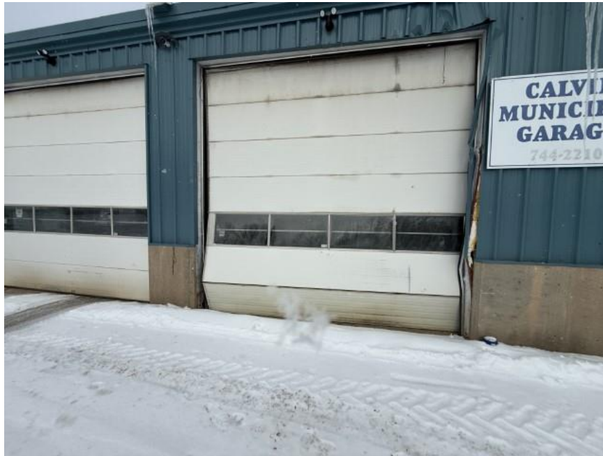
Photo 7: Municipal Garage – Overview of Impact Damage
