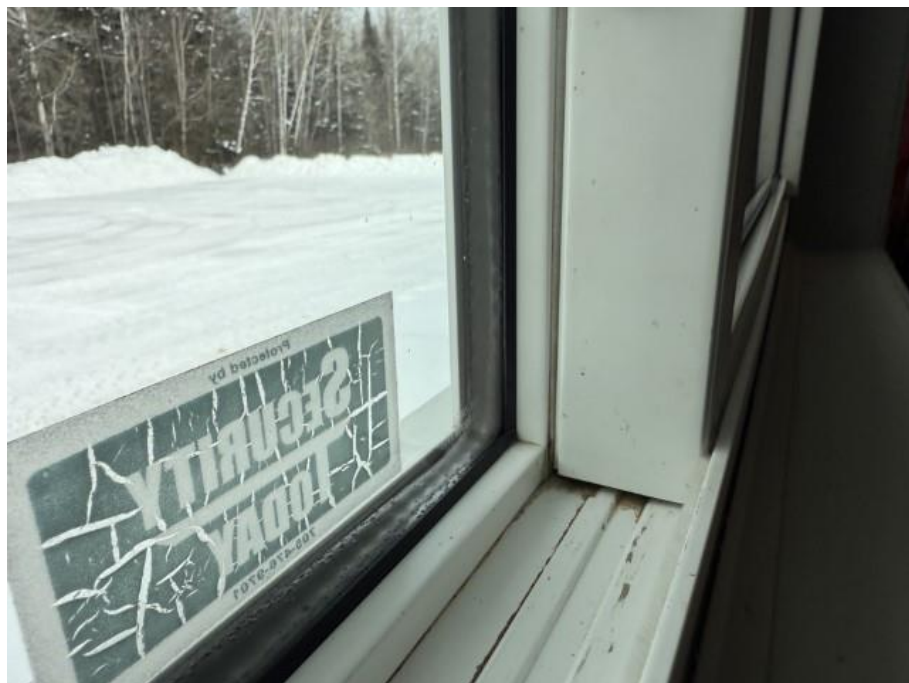
Photo 6: Recreation Hall –Interior Window Condition
