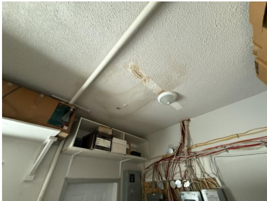
Photo 10: Recreation Hall – Evidence of Roof Leaks
