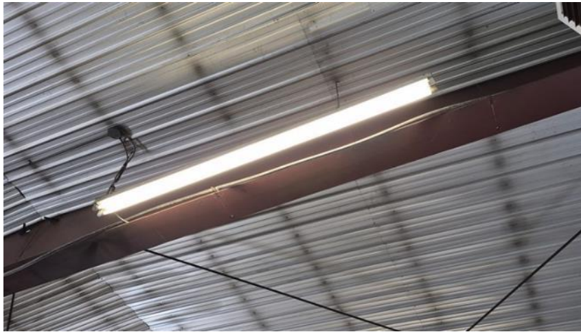
Photo 19: Municipal Garage – Existing Fluorescent Interior Lighting
