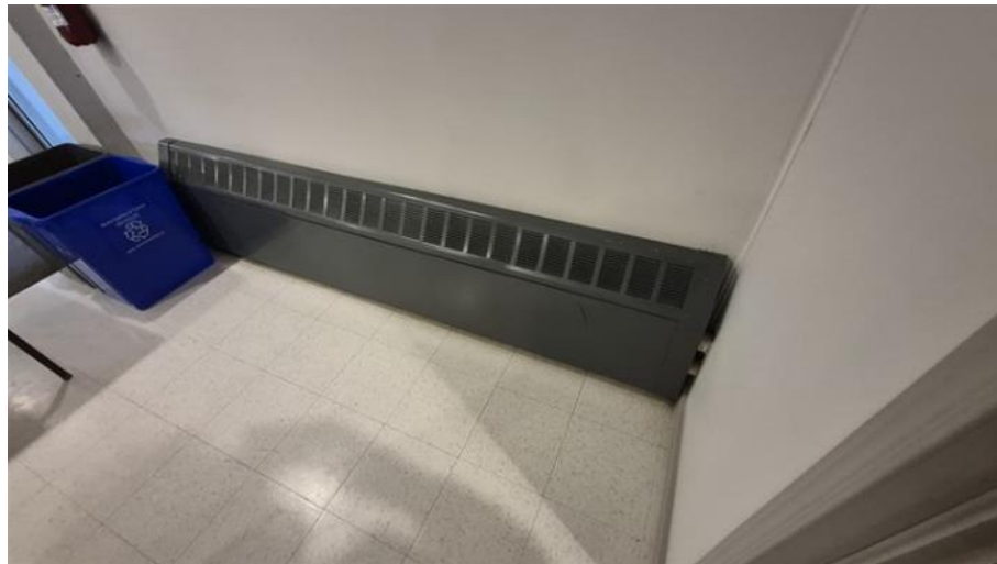
Photo 16: Recreation Hall – Typical Original Fin-Tube Hydronic Heating Convectors
