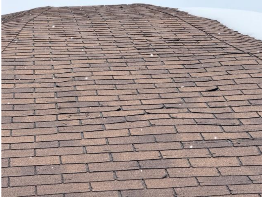
Photo 7: Sand Dome – Severe Asphalt Shingle Deterioration
