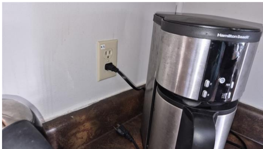
Photo 20: Recreation Hall – Kitchen Power Distribution – Circuit Balancing to permit Multiple Appliance Operation
