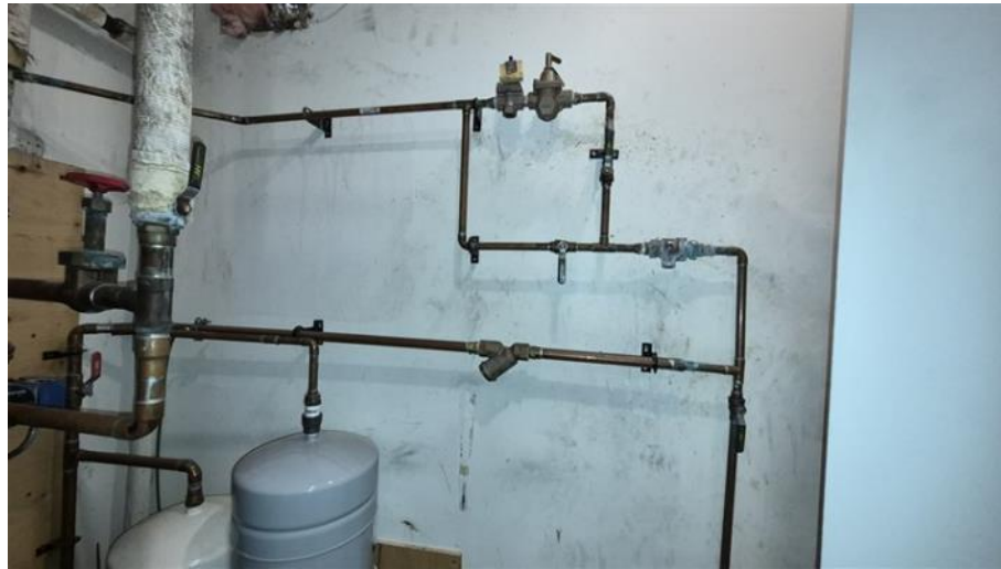
Photo 13: Recreation Hall – Domestic Hot Water Piping Interface to Heating Boiler
