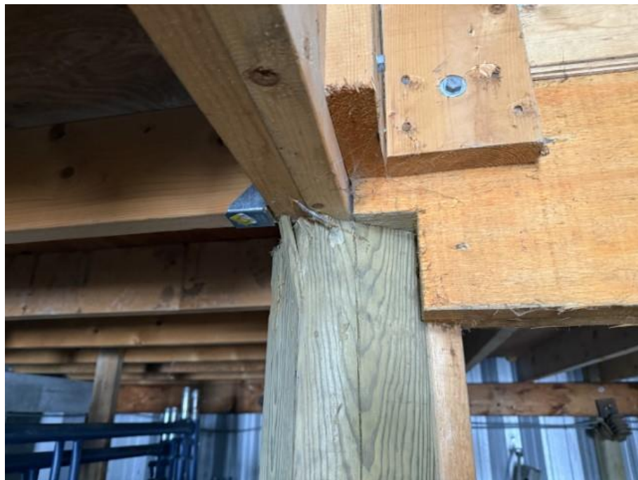
Photo 4: Quonset Hut – Localized Post Displacement
