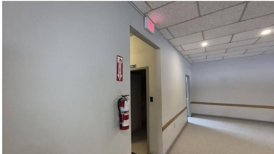
Photo 18: Recreation Hall – Typical Portable Fire Extinguisher
