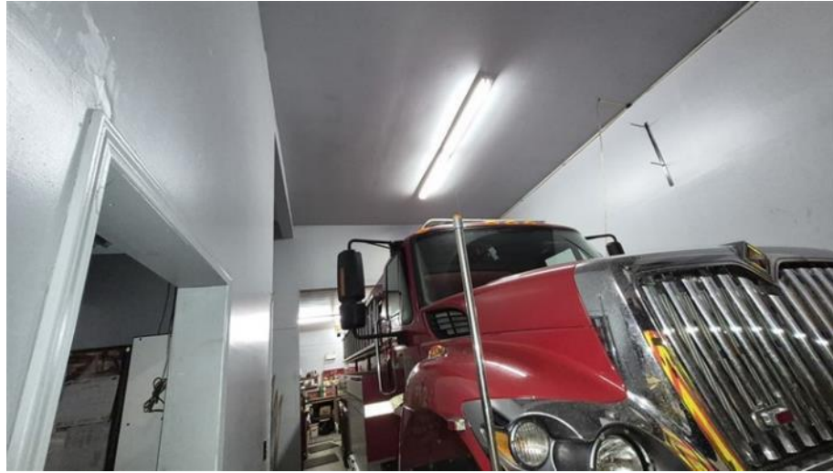
Photo 13: Fire Hall – Typical Existing Fluorescent Lighting
