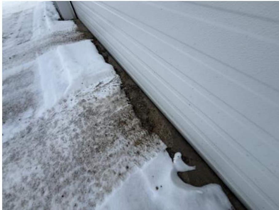
Photo 3: Fire Hall – Slab Spall at Overhead Door
