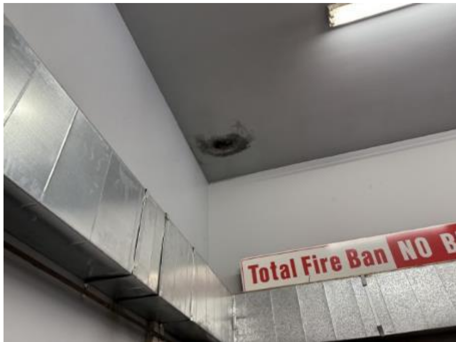
Photo 10: Fire Hall – Stain in Ceiling
