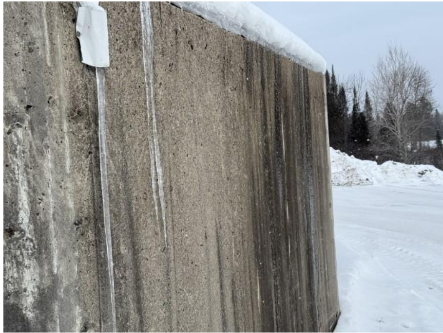
Photo 3: Sand Dome –Concrete Wall Staining
