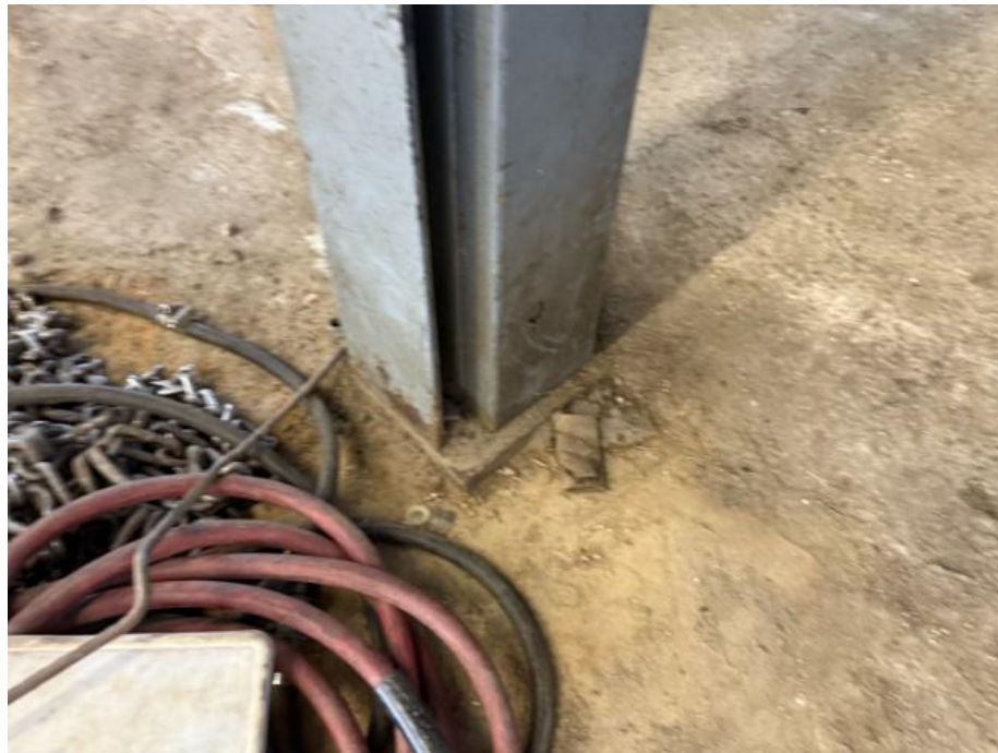
Photo 2: Municipal Garage – Typical Column Base
