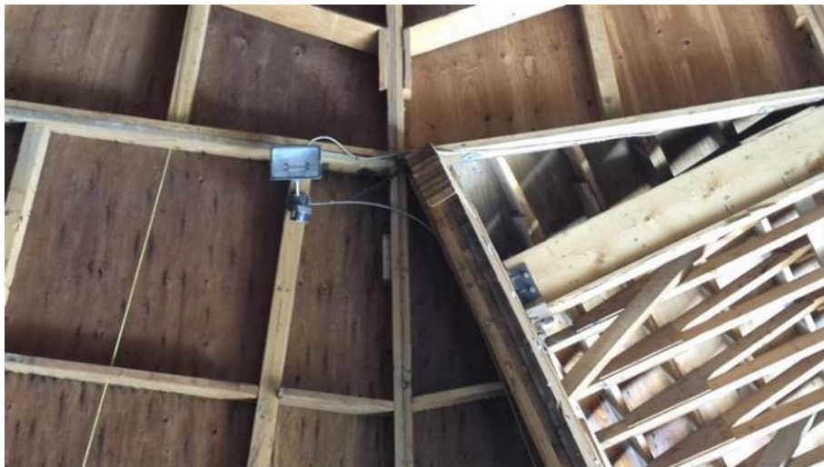
Photo 10: Sand Dome – Non-Functional Interior Light Fixture. Typical of 2
