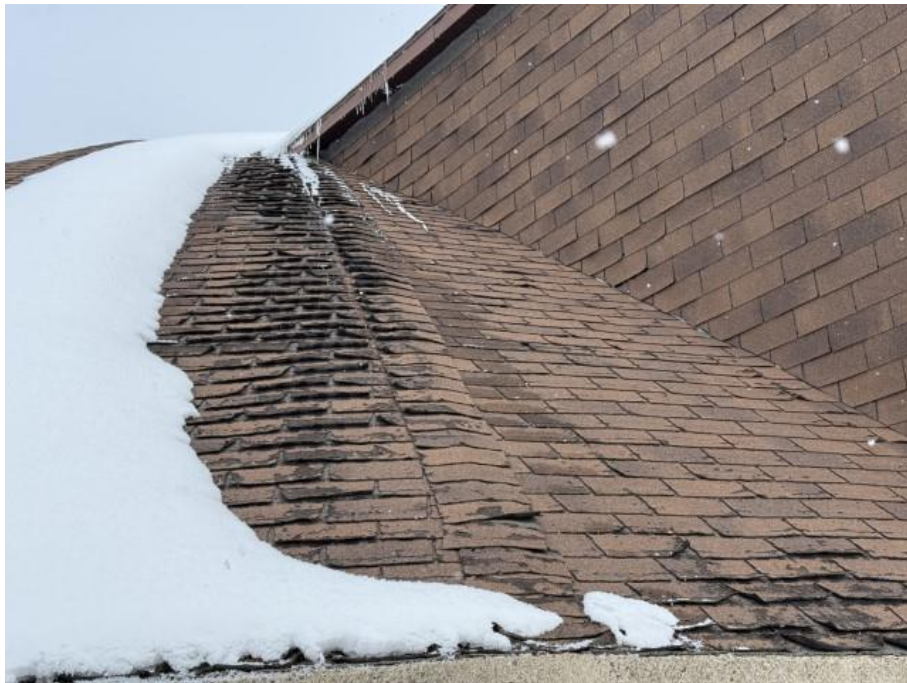
Photo 8: Sand Dome – Severe Shingle Deterioration
