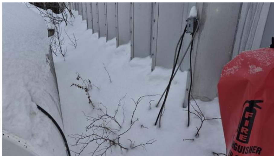
Photo 8: Diesel and Gasoline Tank Dispenser Pump Wiring
