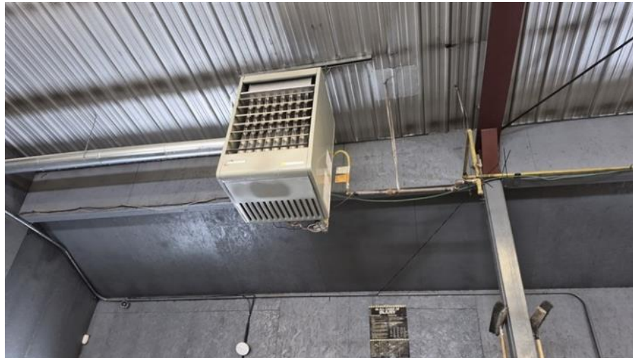
Photo 15: Municipal Garage – Existing Older Garage Area Unit Heater
