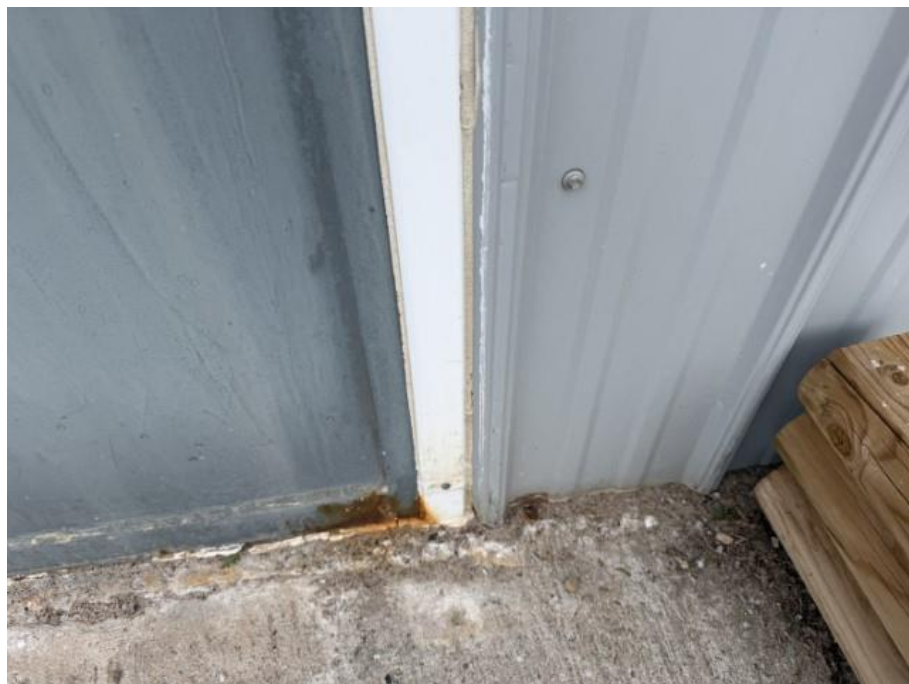
Photo 4: Recreation Hall - Typical Base of Door/Cladding Corrosion
