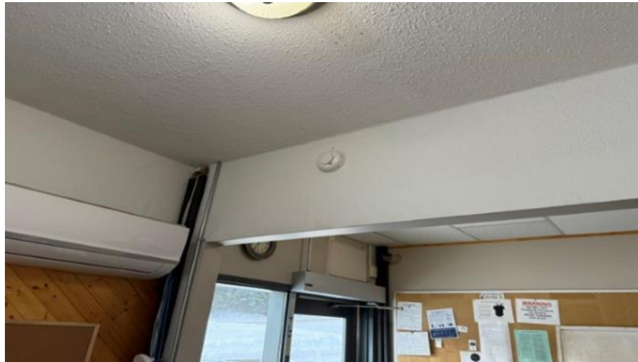
Photo 17: Recreation Hall – Local Smoke Detector. Typical for 2 such Detector Installations
