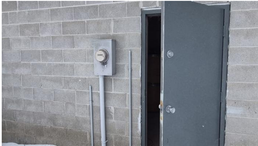
Photo 9: Changing/Storage Building - Electrical Power Service to Recreation Change Room
