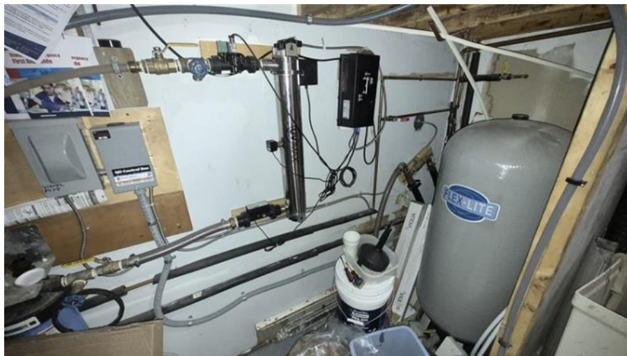
Photo 12: Recreation Hall – Existing UV Water Sterilizer and Associated Plumbing
