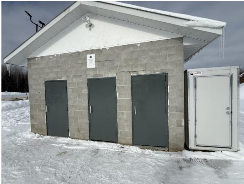
Photo 5: Changing/Storage Building – Doors and Overhead Step Cracking
