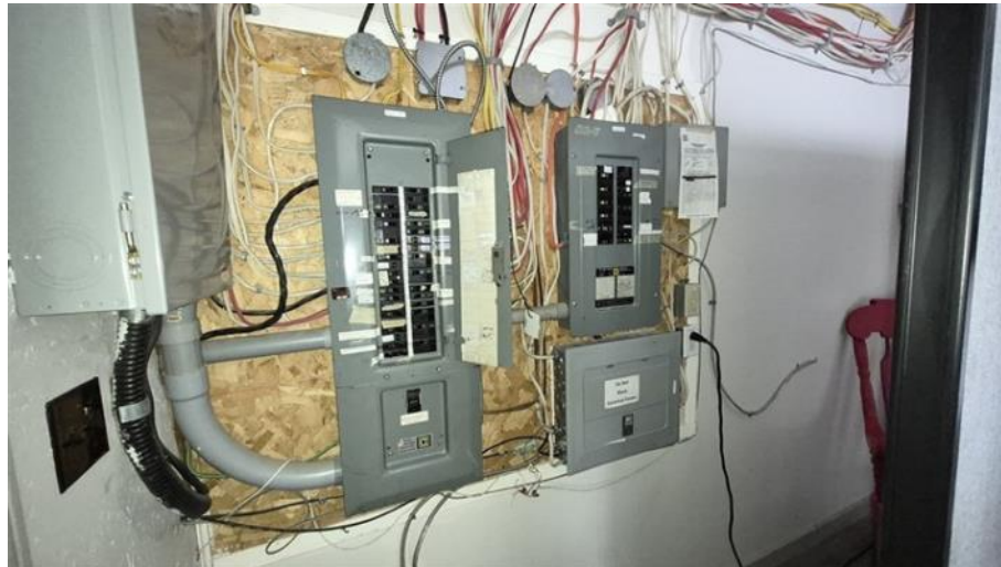
Photo 19: Recreation Hall – Existing Electrical Panels – Circuit Balancing and Identification
