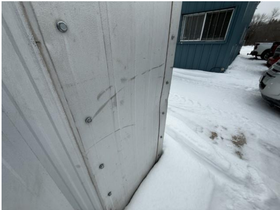
Photo 6: Quonset Hut – Localized siding Damage
