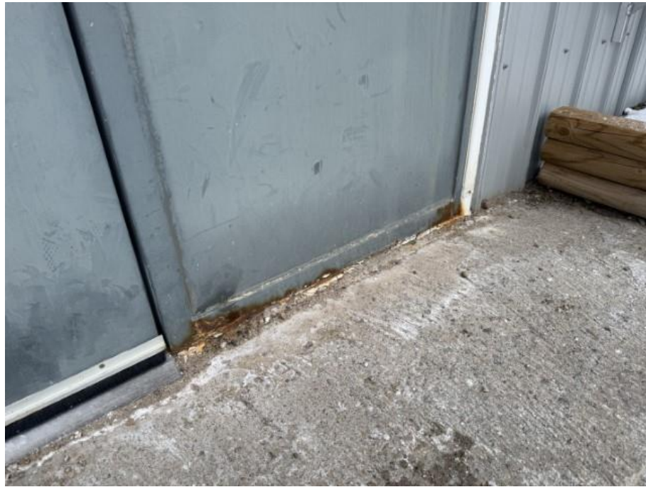
Photo 9: Recreation Hall – Door Base Corrosion
