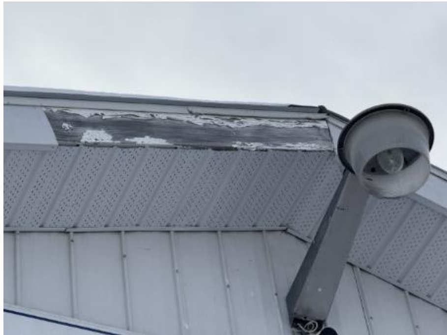
Photo 11: Fire Hall – Unprotected Fascia and existing HID Lighting
