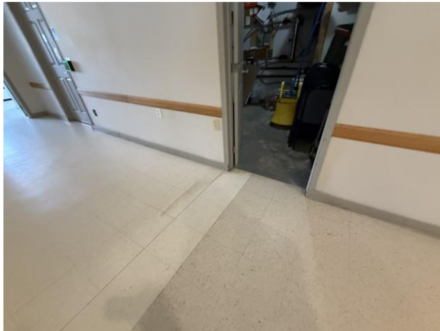
Photo 2: Recreation Hall – Slab-on-Grade Joint Displacement
