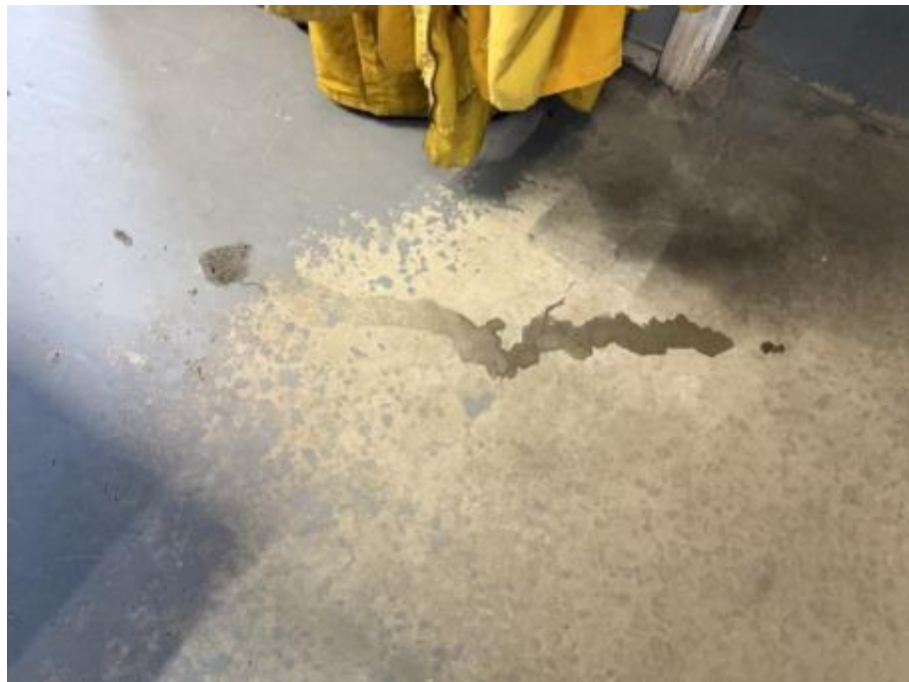
Photo 2: Fire Hall – Slab-on-Grade Cracking
