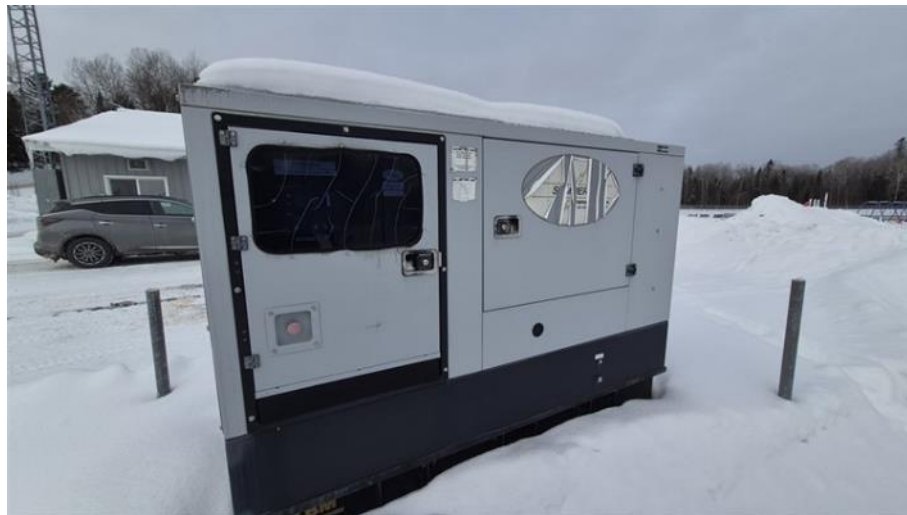
Photo 22: Recreation Hall – Existing Emergency Backup Power Generator
