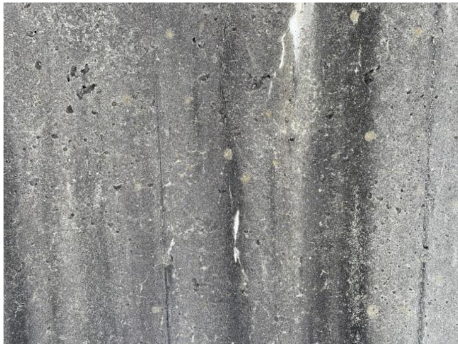
Photo 4: Sand Dome – Concrete Wall Cracking
