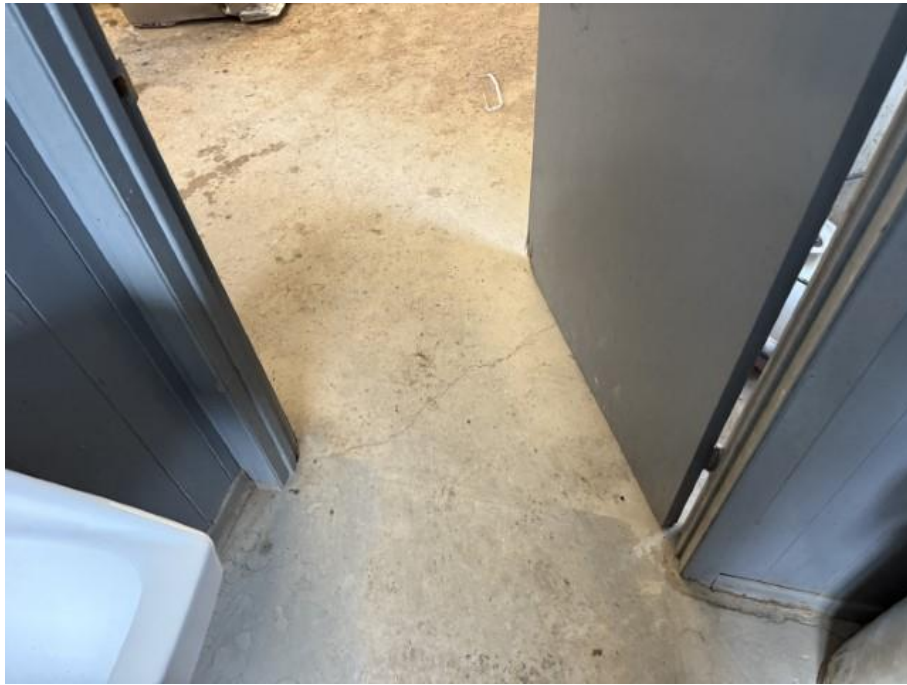
Photo 3: Municipal Garage – Typical Slab Cracking
