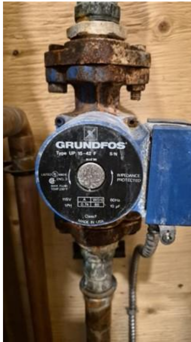
Photo 15: Recreation Hall - Heating Water Circulation Pump
