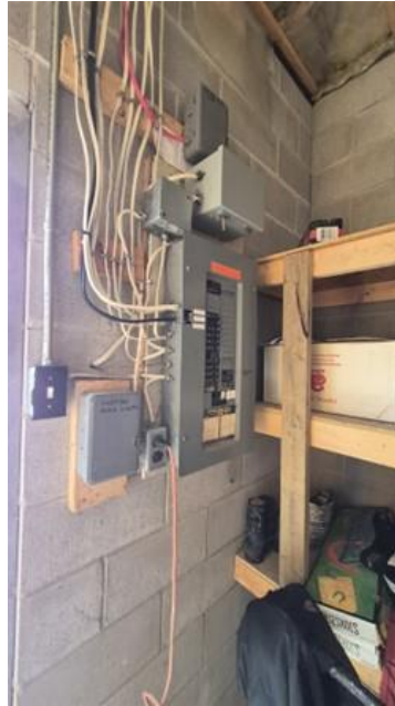
Photo 11: Changing/Storage Building – Electrical Power Distribution and Controls
