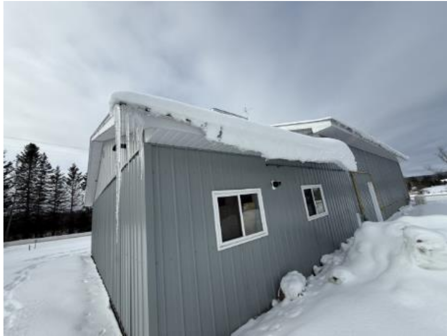
Photo 9: Fire Hall – Snow and Icicle Coverage
