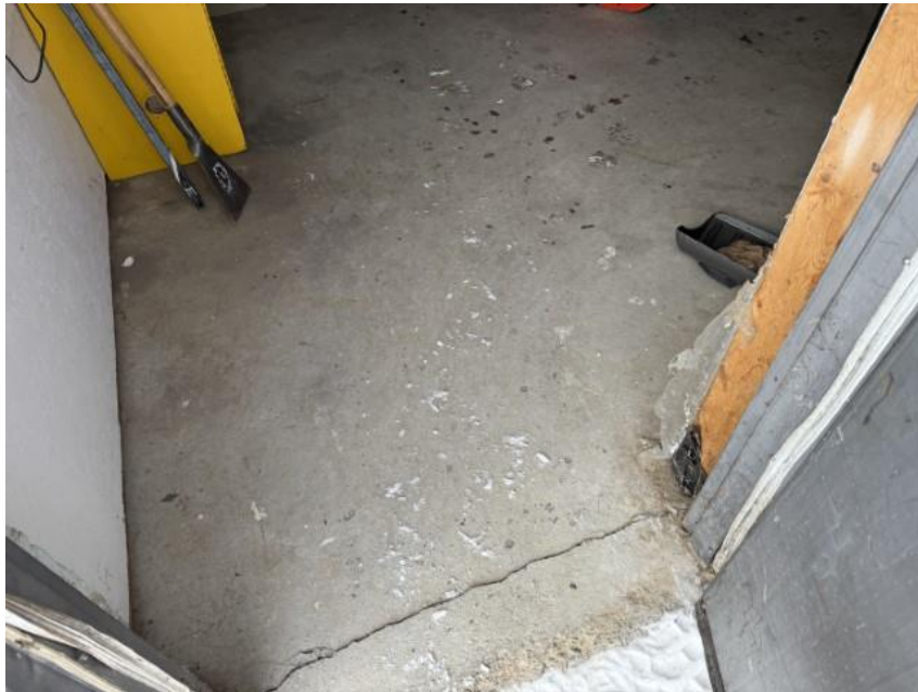
Photo 3: Changing/Storage Building – Cracking at Foundation-Slab
