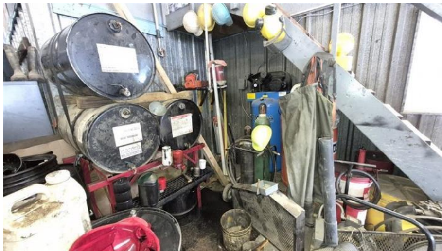
Photo 14: Municipal Garage – Lubricant Storage Obstructing Access to In-Floor Oil Interceptor
