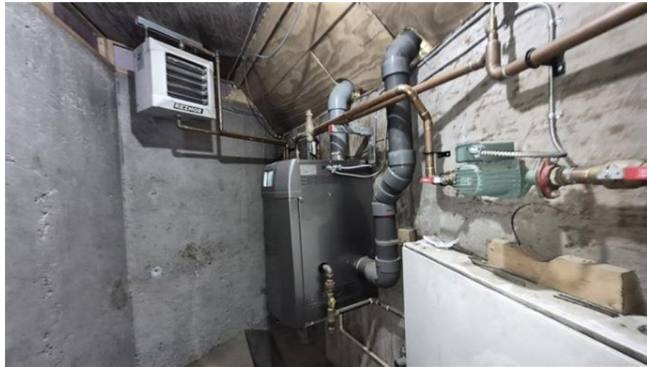
Photo 11: Sand Dome – Existing Heating Boiler and Mechanical Room Heater
