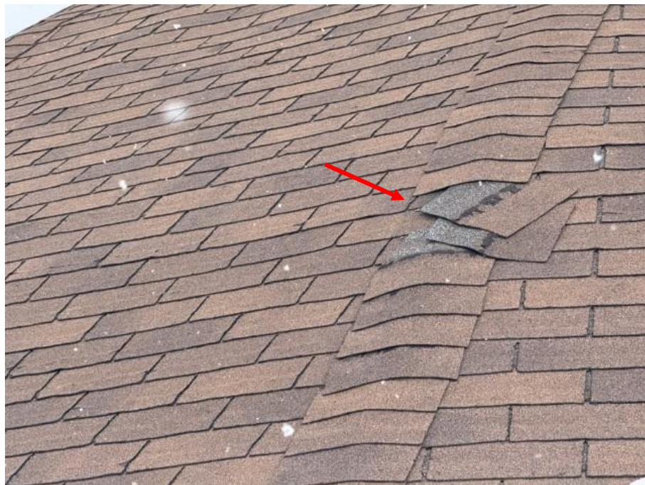
Photo 6: Sand Dome –Localized Shingle Failure
