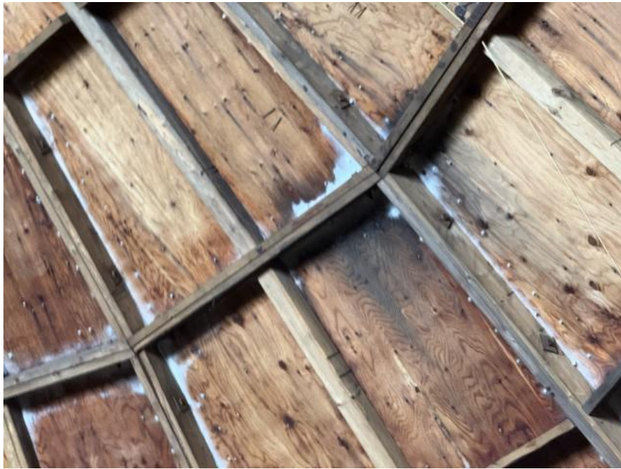
Photo 9: Sand Dome – Localized Sheathing and Framing Moisture Staining
