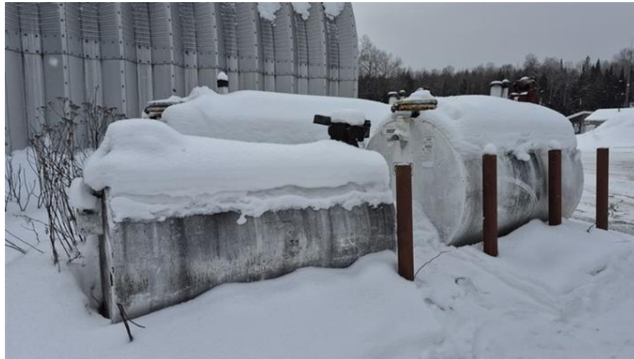
Photo 7: Diesel and Gasoline Bulk Storage Tank Farm
