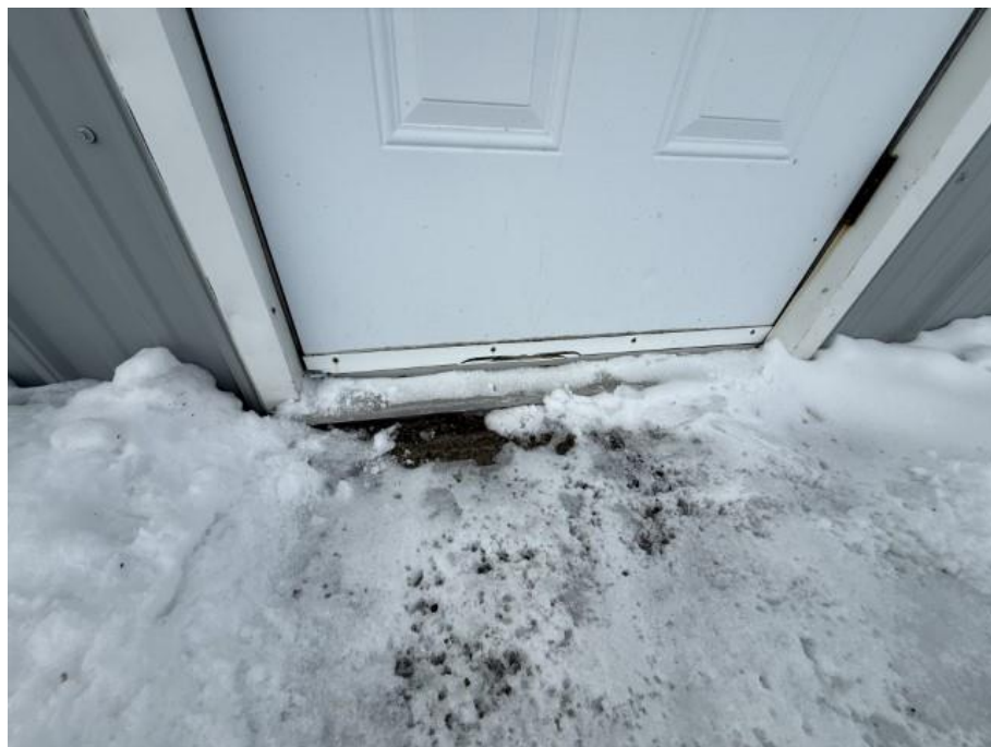
Photo 8: Recreation Hall –Door and Surround Typical Damage
