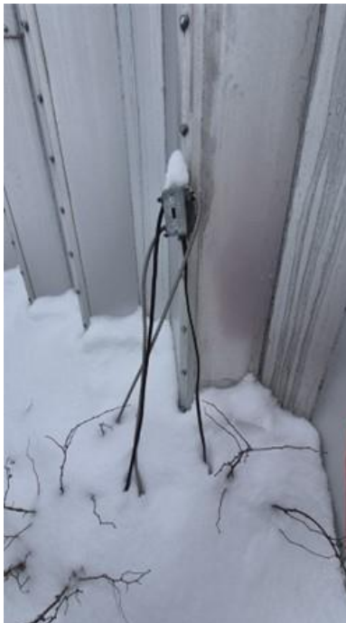
Photo 10: Quonset Hut – Existing Exterior Electrical Wiring
