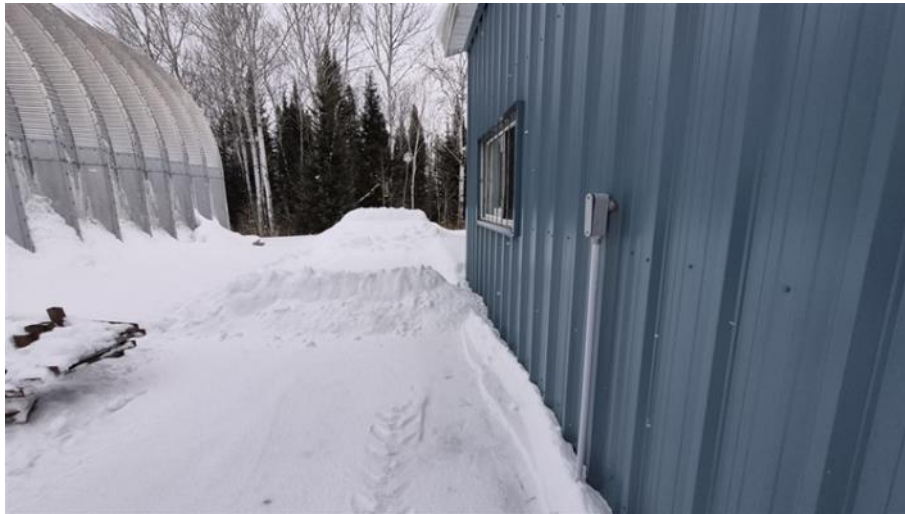
Photo 18: Municipal Garage – Existing Unprotected Power Conduit
