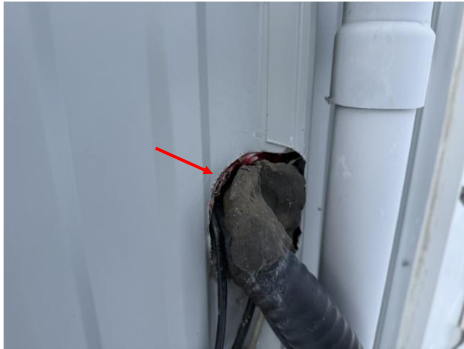
Photo 5: Recreation Hall – Unsealed Exterior Penetration
