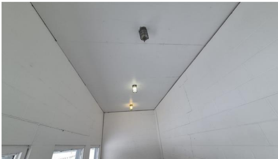
Photo 10: Changing/Storage Building – Changeroom Interior Lighting
