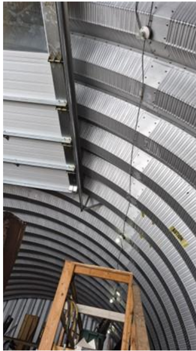
Photo 9: Quonset Hut – Existing Interior Lighting
